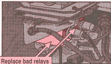
Replace bad relays
